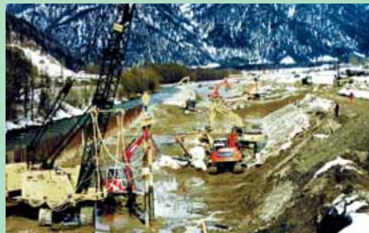
Photos C-3-5: The Großache today. The river bed has been widened and restructured. Construction works under way
