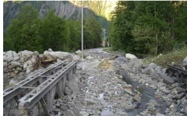
Figure 42: Example of debris deposition on a regional road caused by the outburst of a water pocket of Rochefort glacier (©Autonomous Region of Aosta Valley)
