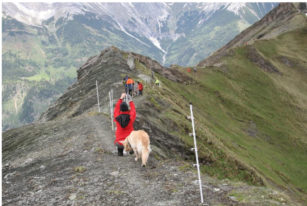
Building the fence at the ridge in the pilot project in Zederhaus/Salzburg. © G. Rauer
