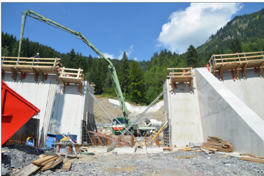
Fig. 10: Realisation of a debris flow control structure in the torrent Zillenbach, municipality Hindelang, Oberallgäu (Picture: WWA Kempten)
