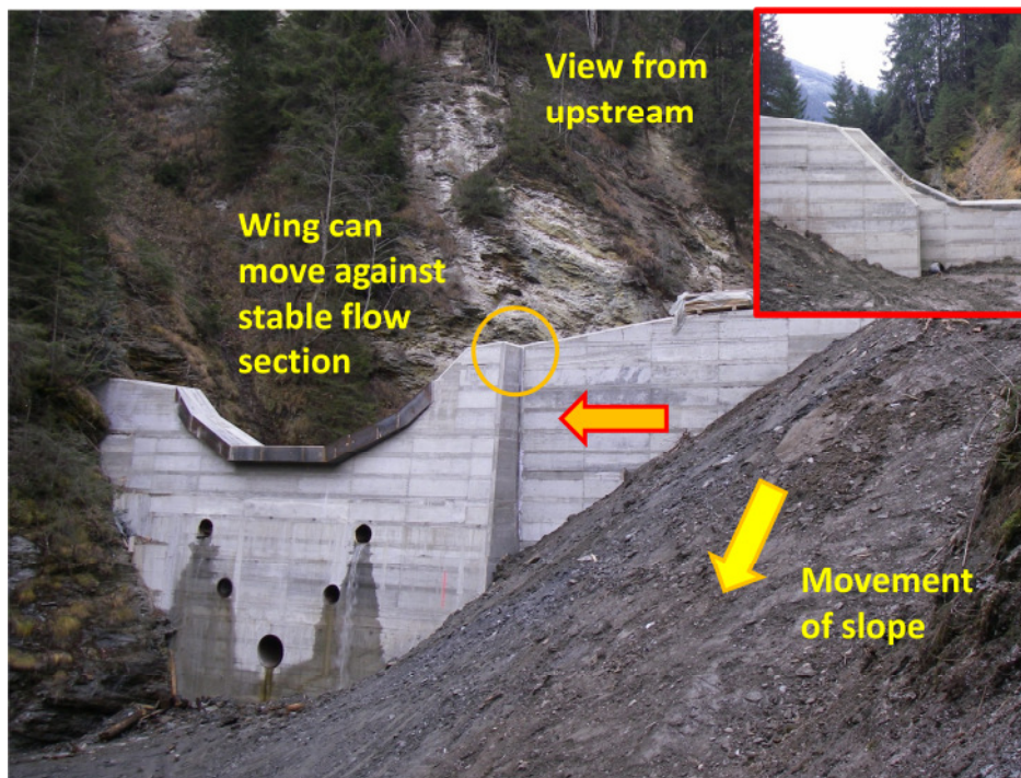
Check dam with a slidable wing to balance lateral mountain pressure, Source: die.wildbach (Salzburg)
