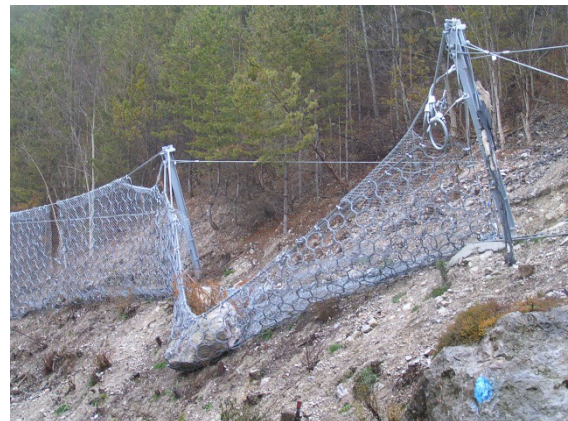
Fig. 11: Monitoring is essential to detect the necessity of maintenance and as a consequence to keep up functionality
