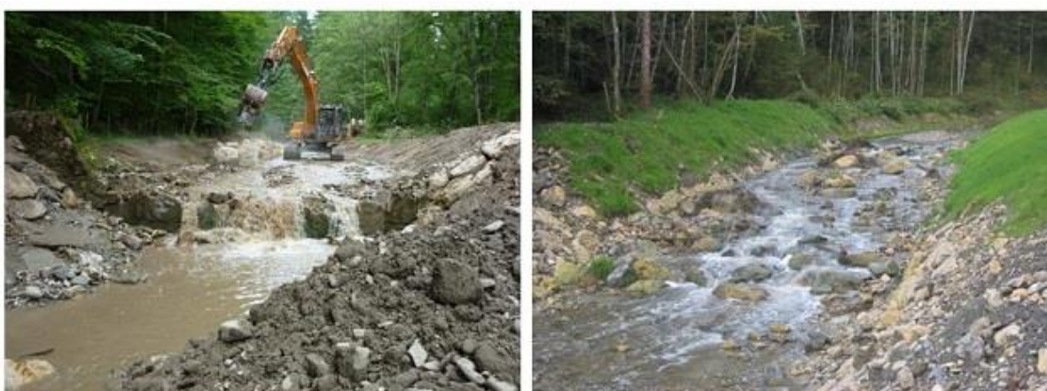
Figure 13: During and after the reconstruction (ramp with a height of 1.6 m and a length of 70 m)
