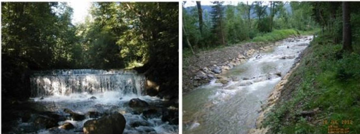
Figure 12: Before and after; a 3 m high check dam is replaced by a 120 m long ramp
