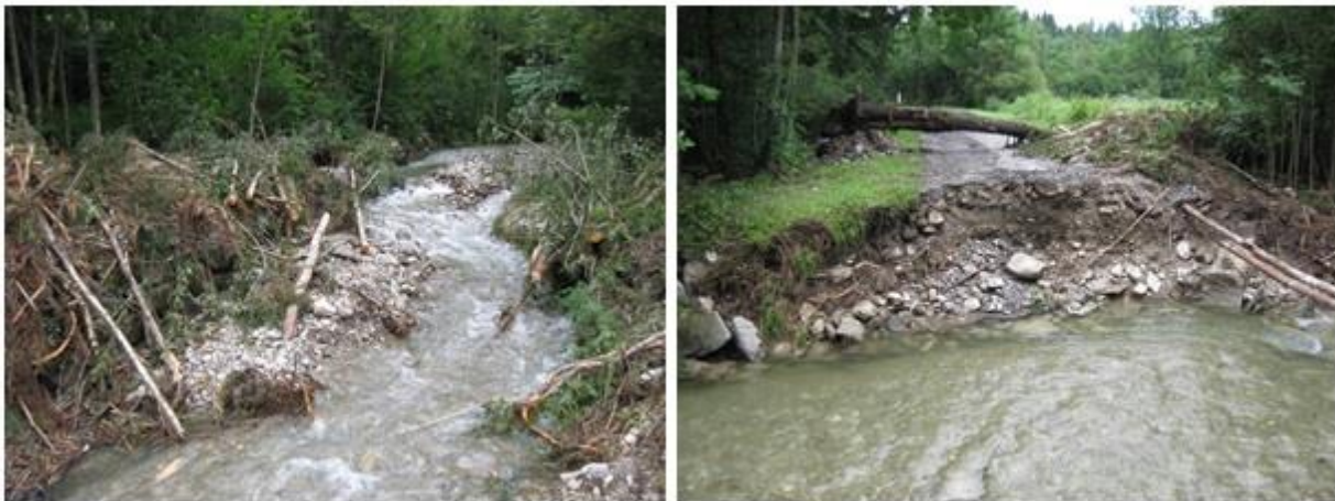
Figure 11: Wood log jam destroyed a bridge; also several check dams are damaged
