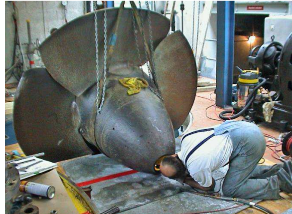
Figure 5: Employment creation for the green industry: Here during the revision of the hydro-power station of Luterbach in Switzerland (320kW) (© Hydroelectra AG 11 )
