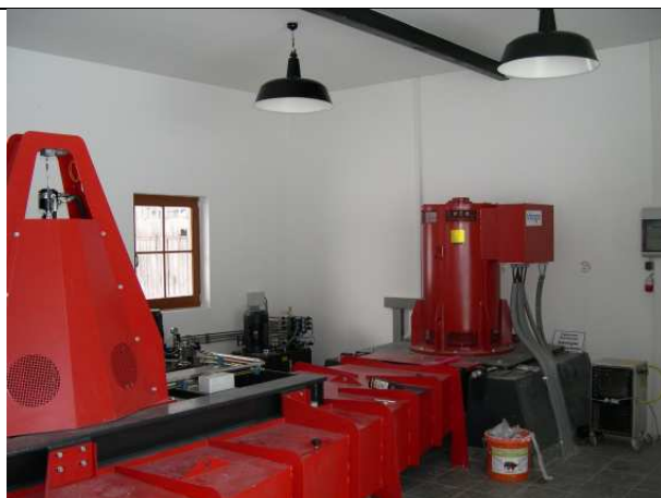
Figure 5: Power station SHPP Cumberland © Herzog von Cumberlandstiftung
