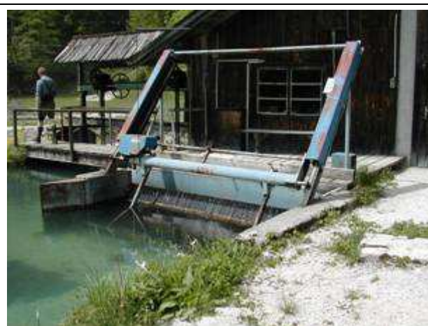
Figure 6: Weir system SHPP Cumberland © Herzog von Cumberlandstiftung
