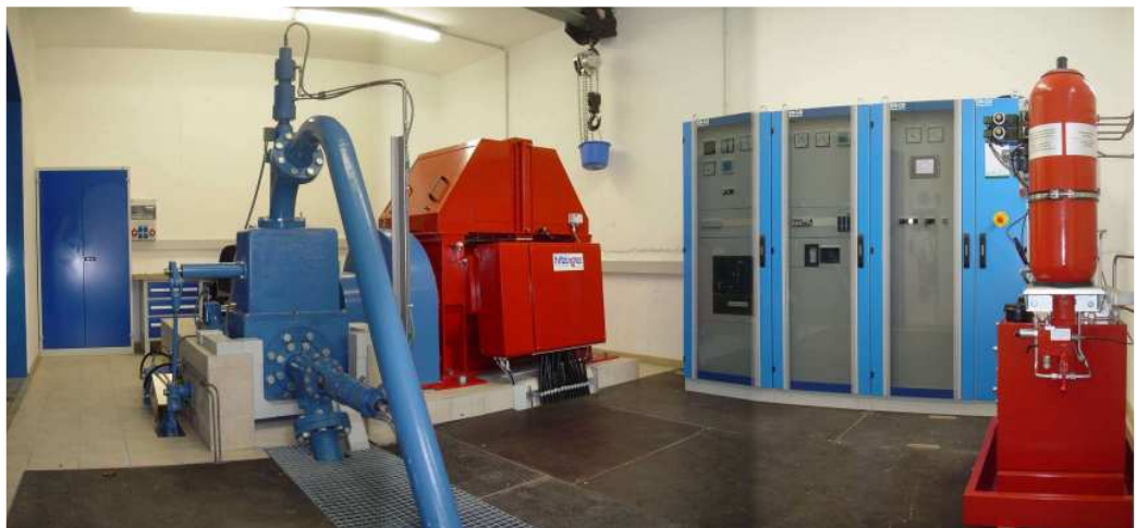
Figure 23: Interior panorama (Hydroelectric generating set with Pelton turbine, synchronous alternator and electrical equipment) © Gemeindewerke Garmisch-Partenkirchen
