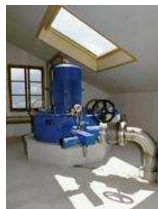
Figure 44: 75 kW power group. © MHyLab
