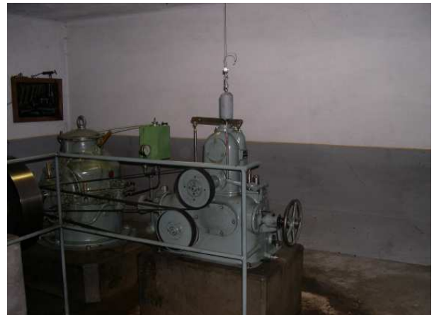
Figure 4: Power station SHPP Magerlmühle © Christoph Wagner
